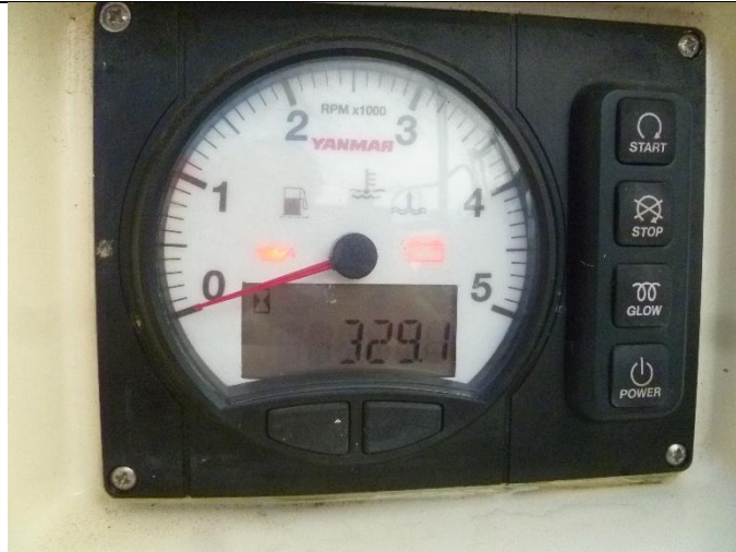
Engine monitoring & switch panel.
